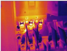
Electronic and electrical testing
